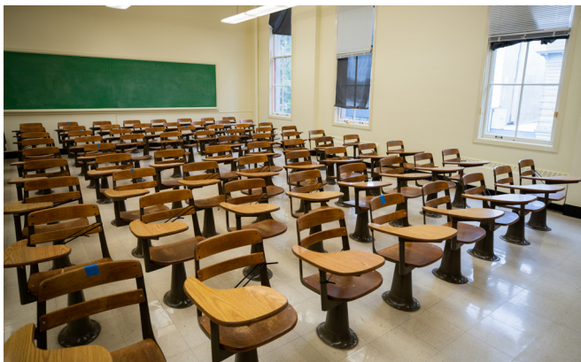
Classrooms contain immovable seating with inadequate desk, seat, and aisle size. As a result of inadequate classroom space and function, learning and instruction has been forced to move, where space allows, into the hallways, stairway landing areas, and faculty offices.
