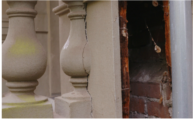
Water infiltration behind the historic façade is exacerbating the deterioration of the historical elements.
