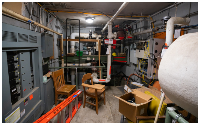
The mechanical and network rooms are insufficient in size and contain obsolete equipment, asbestos piping, and infrastructure operating well beyond its useful life. The mechanics of the building spill out into common space with asbestos and exposed piping and wiring.
