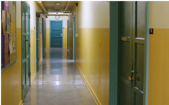
Doorways lack adequate height and necessary width for ADA accessibility. The narrow, tight spaces and ADA inaccessibility is consistent throughout the buildings, in stairways, bathrooms, elevators, and lobby spaces.
