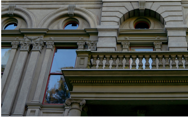
The historic buildings are severely seismically deficient and constructed with unreinforced masonry that will fail and collapse in a Cascadia earthquake.
