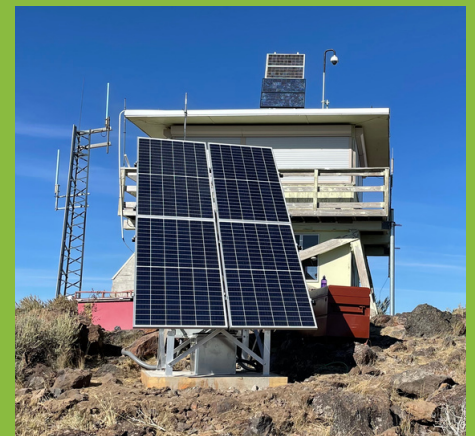
An example of a fire camera (top of building) and seismic sensor (right of image) located at the defunct Wagontire Mtn Lookout Tower in Harney County.
